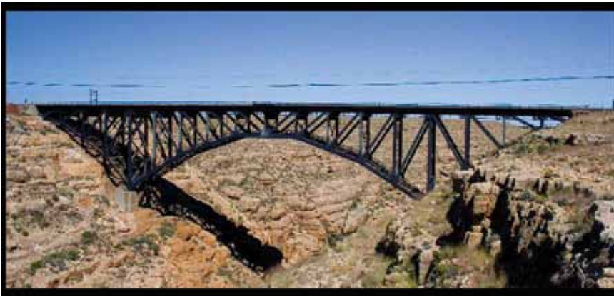
Diablo Canyon Bridge 2012 Here is the same bridge over Diablo Canyon as it appears today, in northeastern Arizona and not far from the author's backwoods home.
